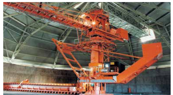
Circular Stockyard with Cantilever Reclaimer
