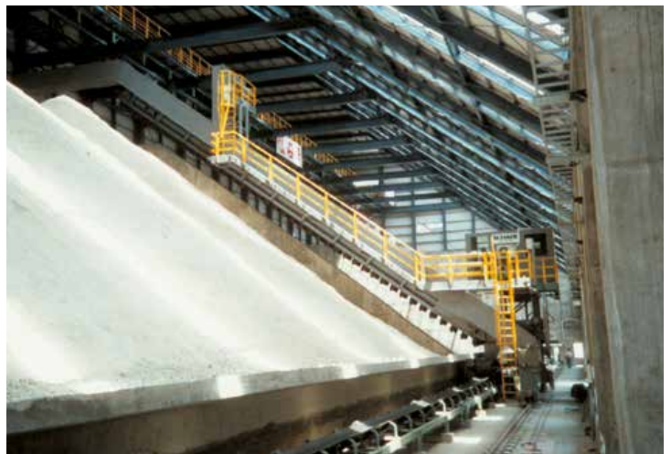
Semi-portal Scraper Reclaimer
